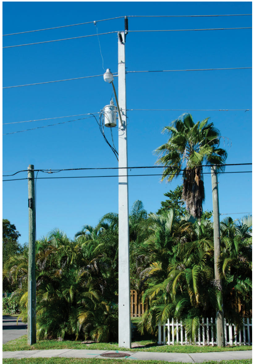
This photo shows an FPL concrete pole, an example of the company's efforts to make the energy grid stronger and more storm-resilient, flanked by two older wooden poles. FPL cannot remove the wooden poles until other utilities transfer their equipment to the cement pole.
