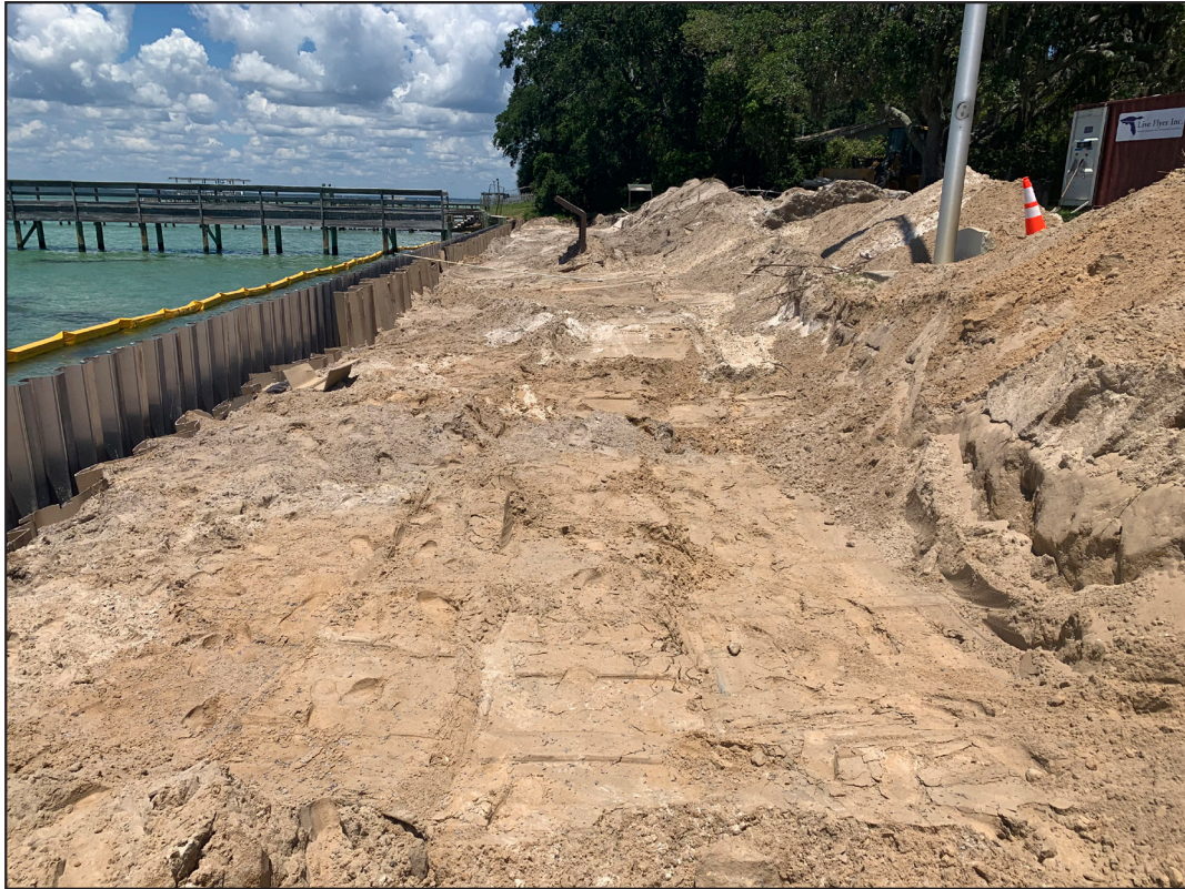
Figure 7. View of dirt pulled back from seawall during seawall construction, facing northeast.
