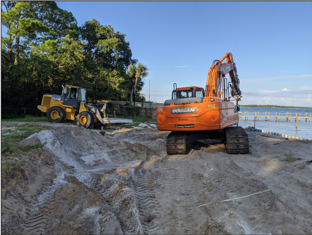
Figure 5. View of heavy equipment used by Live Flyers, Inc. during seawall construction.
