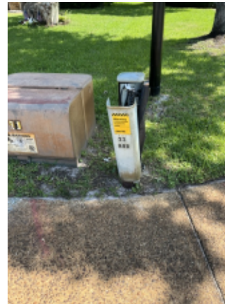
Telephone box 3799 Misty Way, (HBB 22)
