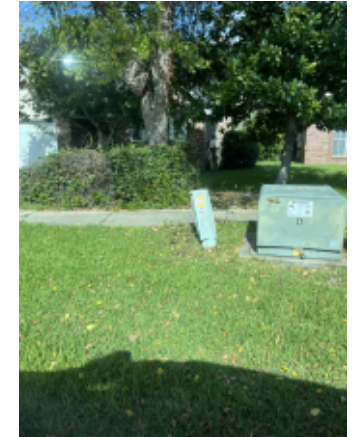
Telephone box 3770 Misty Way (HBB 5)
