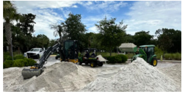
ABOVE DPRD Equipment (Source: The Destin Log)
