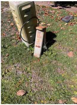
Telephone Cable Box 2 QW – 1110 Quail Circle
