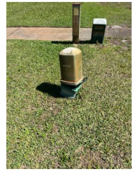
TV Cable Box 1212 Quail Wood Drive
