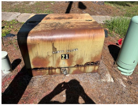
FPL Power Box 21 1106/08 Quail Circle Excessive Rust
