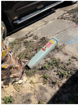
Broken Telephone Box HBB-8
