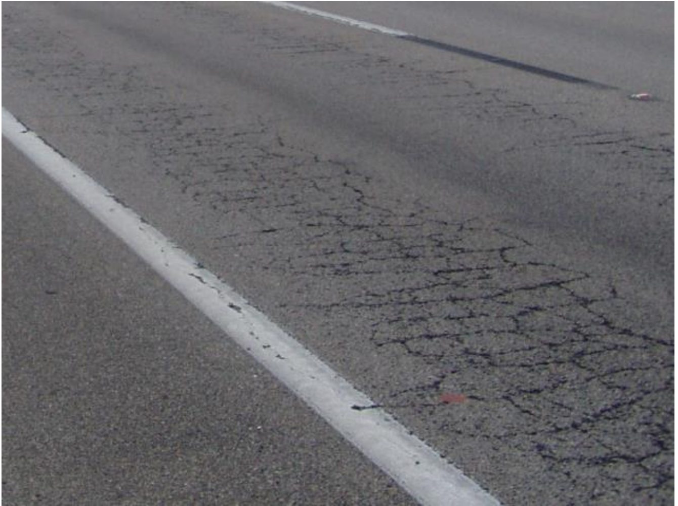
FIGURE 10. CLASS III CRACKING
