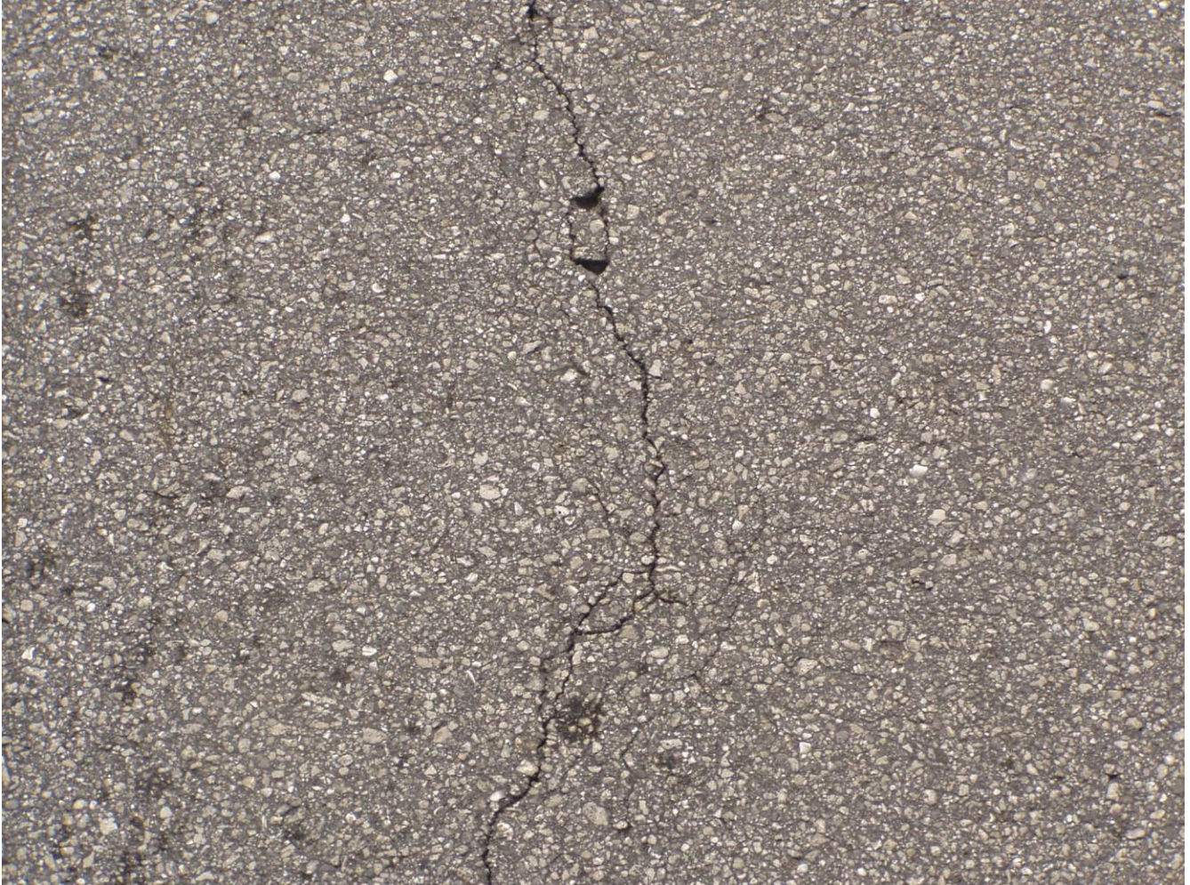
FIGURE 9. CLASS II CRACKING
