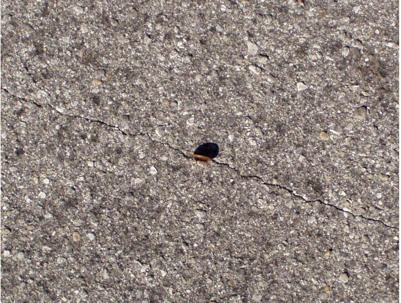
FIGURE 8. CLASS I CRACKING
