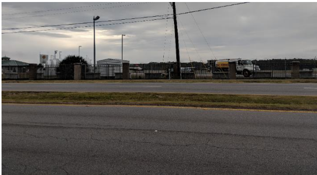
Figure 6 - Pavement surface deterioration and lack of high friction surface
