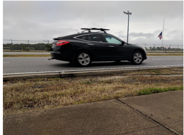
Figure 2 - Excessive drop off at curbing
