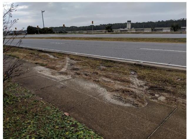
Figure 4 – Excessive Vehicle Runoffs
