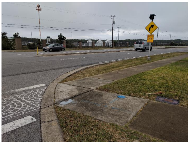
Figure 1 - Sidewalks and crosswalks not meeting standards
