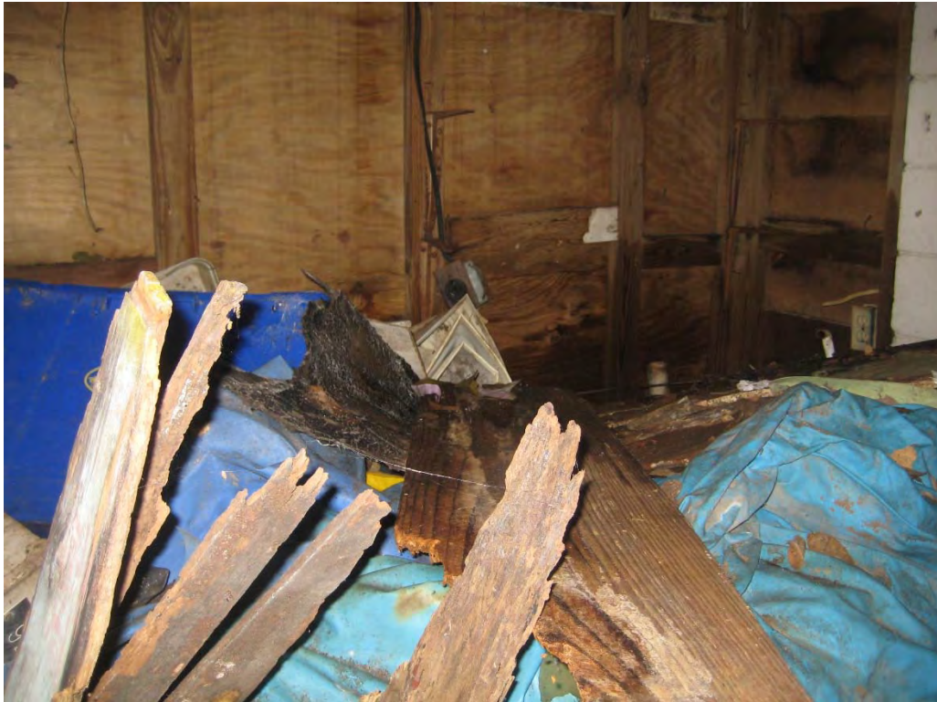
Photo 21 View of interior of structure showing much residential debris
