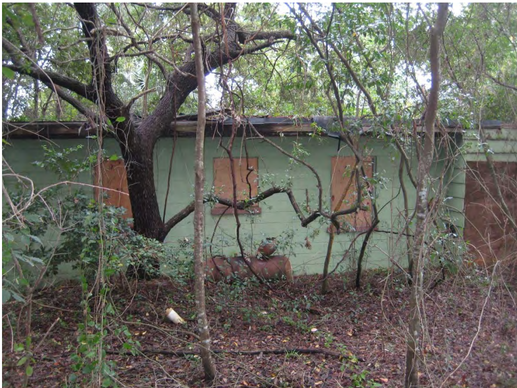
Photo 16 View of residential structure, east elevation with view of natural gas cylinder along wall
