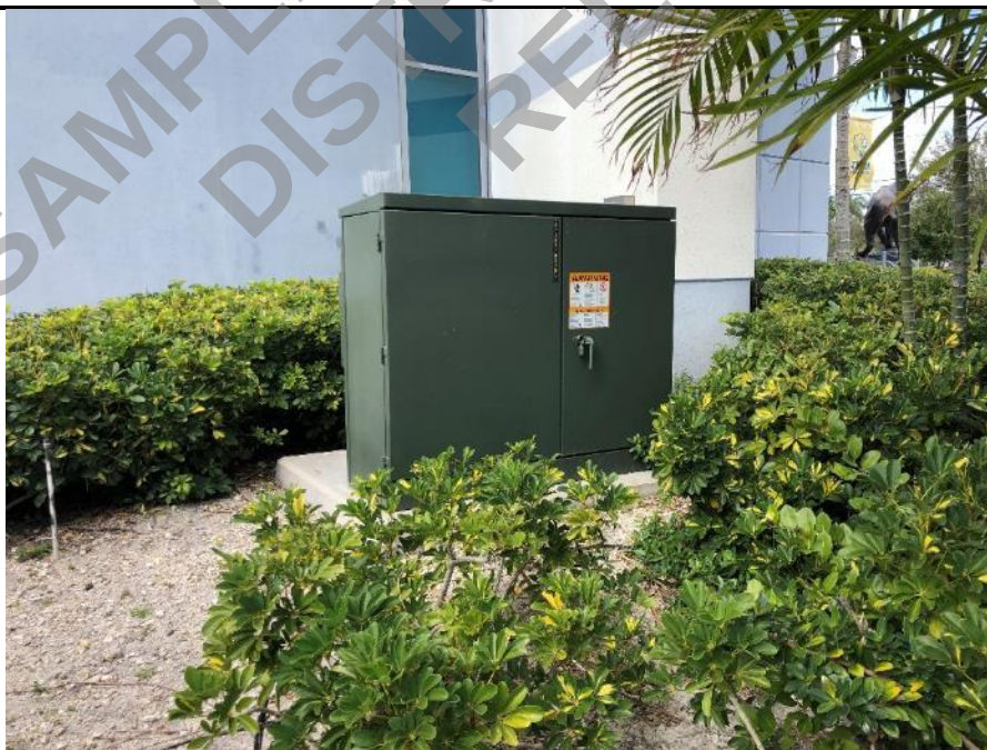
Photo 31: Transformer provided by Florida Power and Light.
