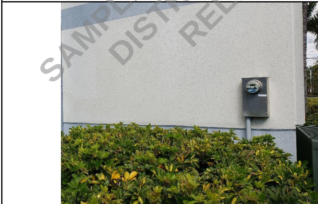
Photo 88: Electric meter located on building exterior.
