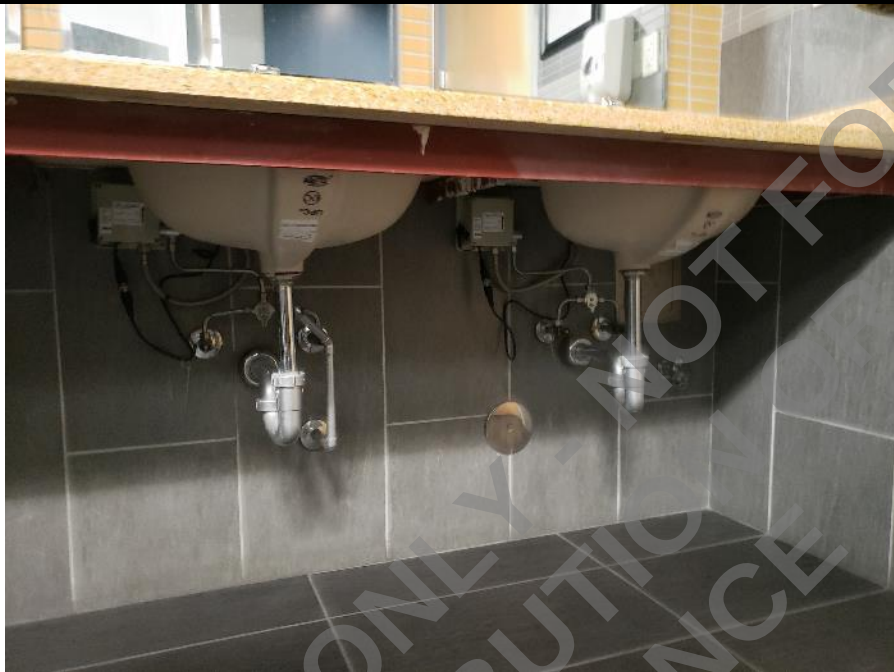
Photo 81: Typical plumbing fixtures with automated faucets
