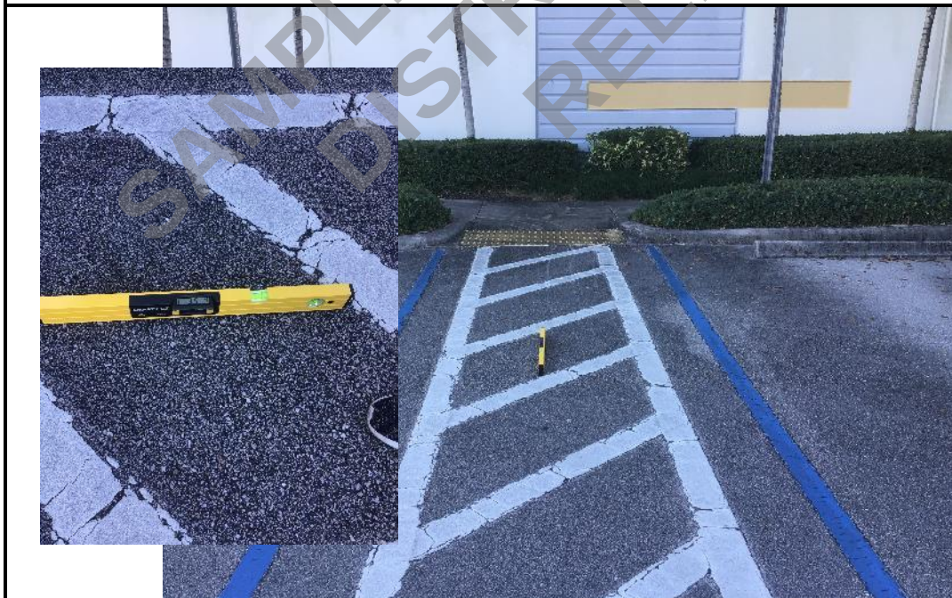
Photo 124: Running slope of access aisle obtained was 3.5% which exceeds maximum allowable of 2.08%.
