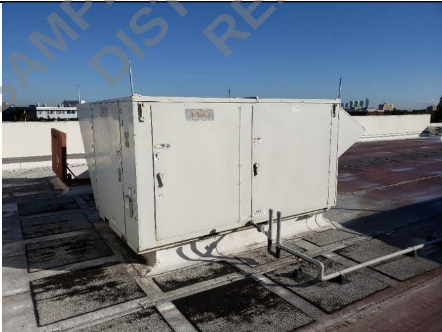
Photo 76: Typical view of roof mounted HVAC.
