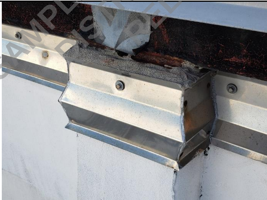
Photo 65: Cracked sealants at surface mounted counter flashing.
