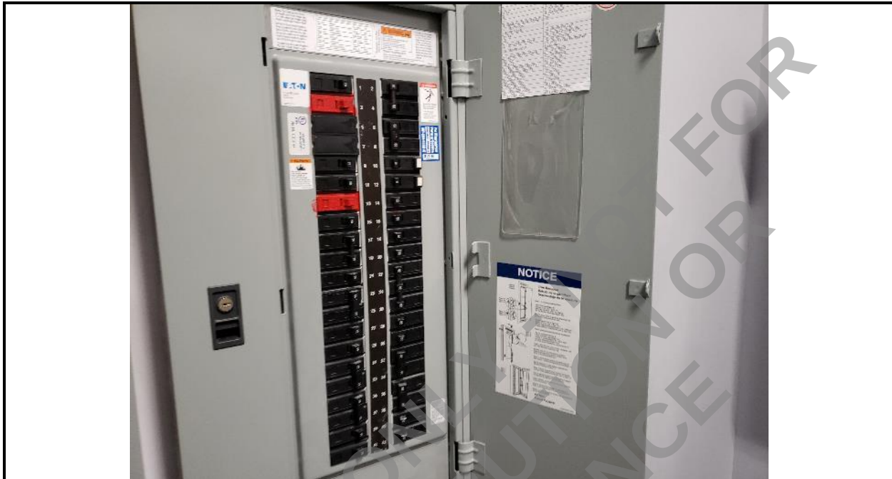
Photo 87: Typical electrical panels observed on site.
