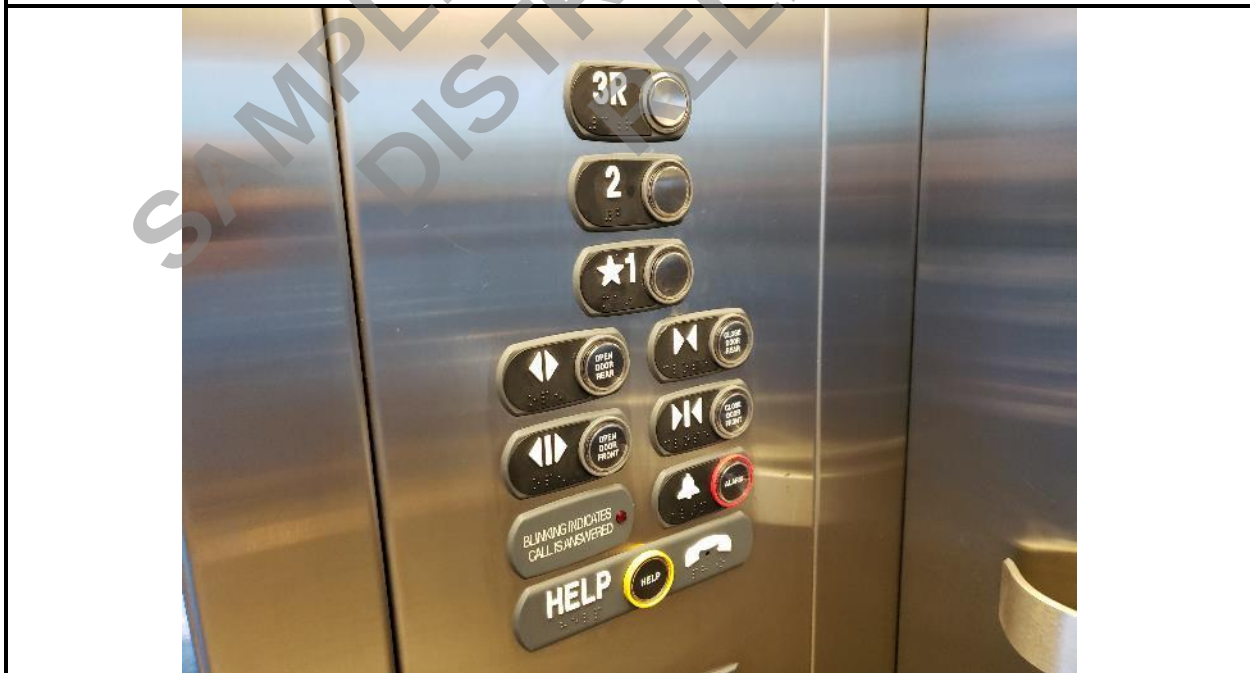
Photo 94: Elevator interior control panel.
