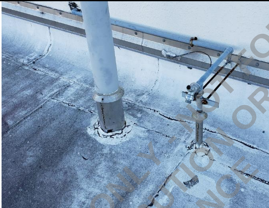
Photo 64: Cracked and deteriorated liquid flashing at penetrations.
