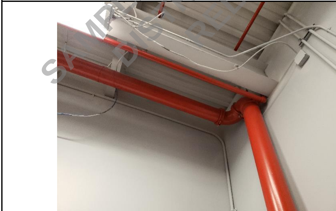
Photo 100: Fire suppression system risers.
