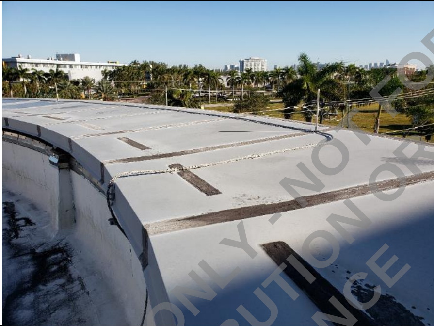
Photo 66: Deteriorated flashing at coping cap.
