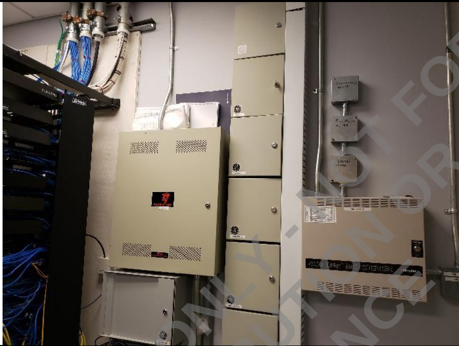
Photo 101: Fire alarm control panel.
