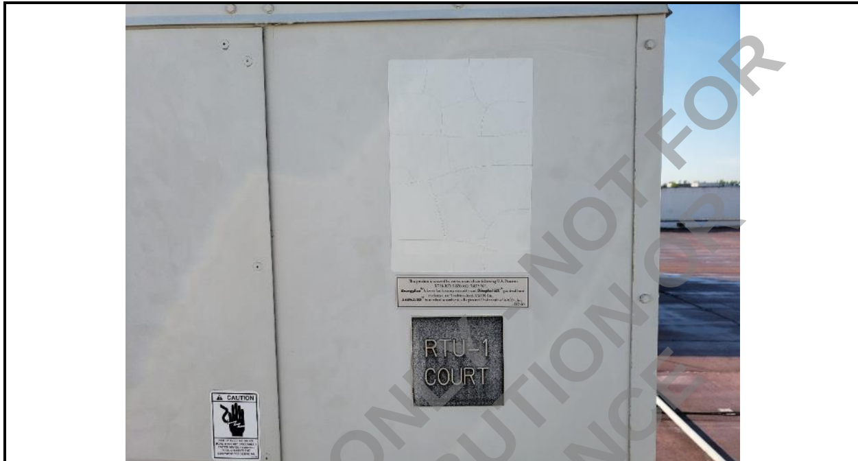
Photo 79: Identification labels faded/not visible on most RTUs.
