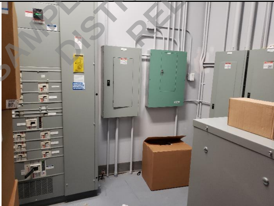
Photo 86: Main electrical room located on first floor
