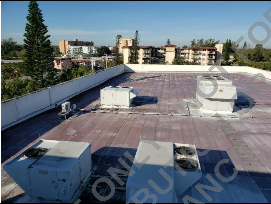
Photo 75: Typical view of roof mounted HVAC.
