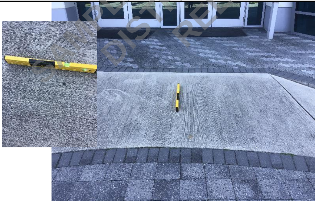
Photo 118: Running slope at main entrance ramp at east elevation being obtained. Measurement was observed to be 9.7%, which exceeds the maximum allowable of 8.3%.
