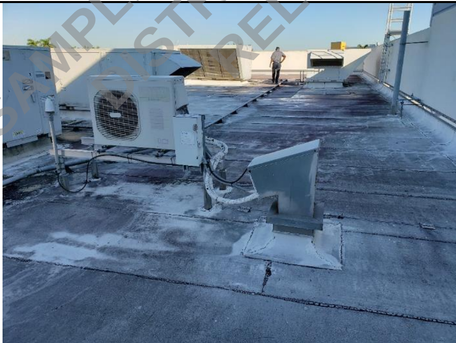
Photo 78: Roof mounted split system air conditioner.
