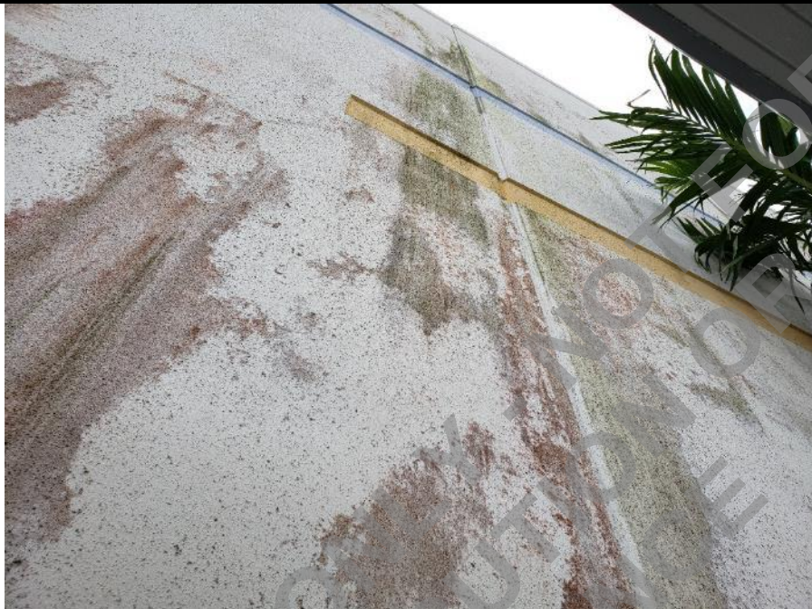
Photo 42: Deteriorating paint on exterior walls.
