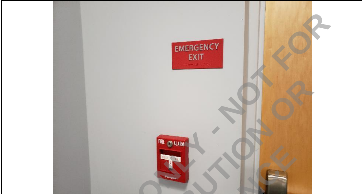
Photo 97: Audible fire alarm.
