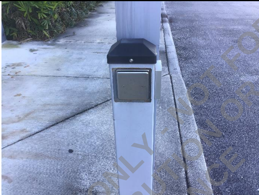
Photo 115: Automatic door opener at north entrance.
