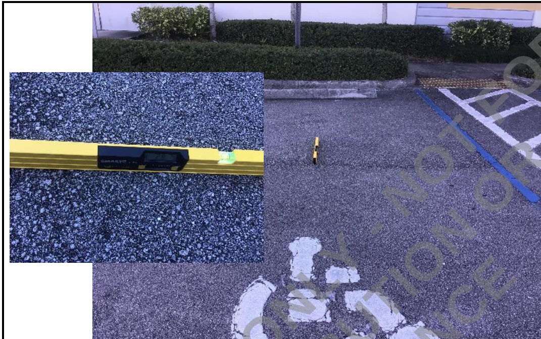
Photo 123: Running slope measurement obtained of left parking spot was 2.8% which exceeds the maximum allowable of 2.08%.
