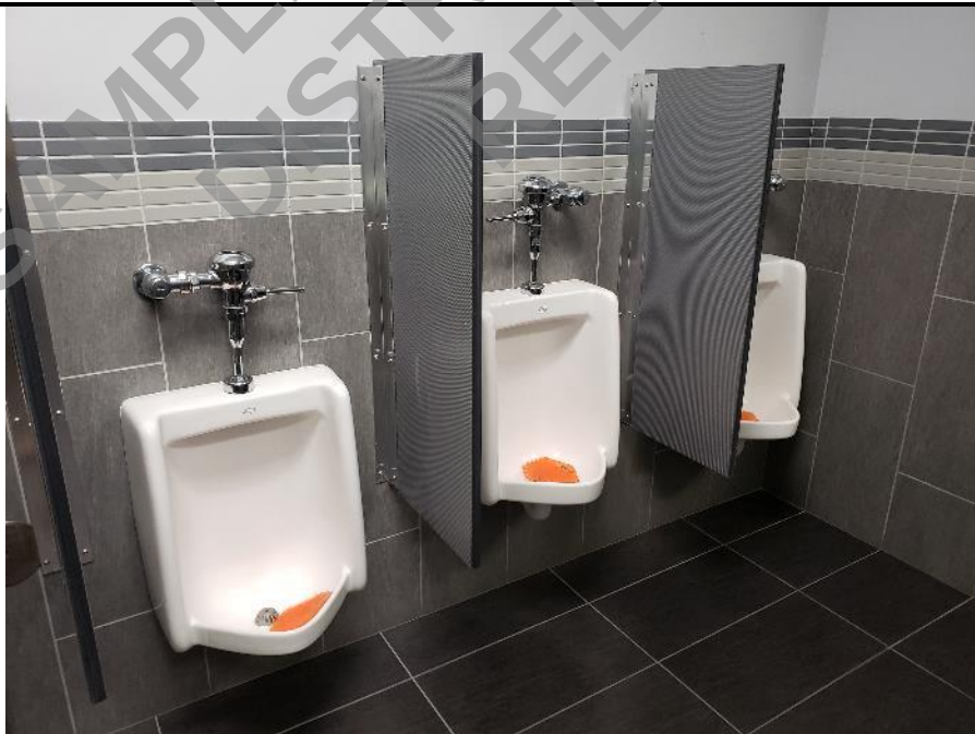
Photo 82: Typical plumbing fixtures in restrooms.
