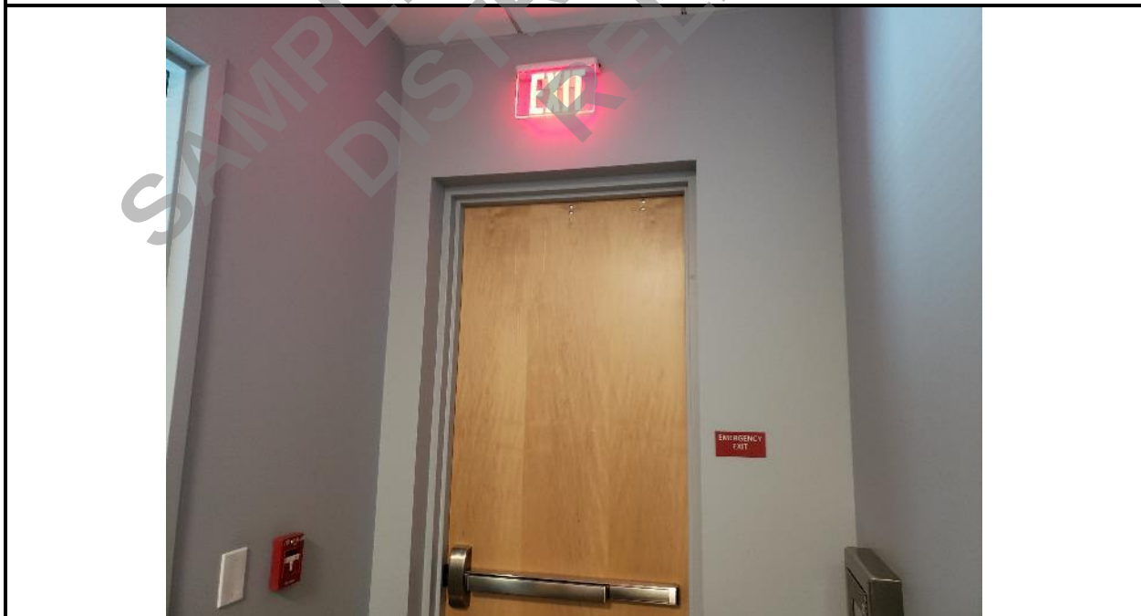
Photo 98: Lighted exit signs.
