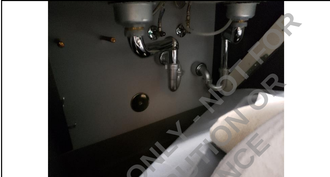
Photo 83: Typical plumbing fixtures in common area sinks.
