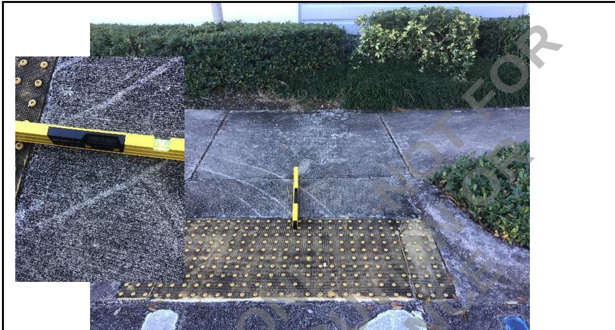
Photo 125: Running slope of ramp at access aisle exceeds maximum allowable for 8.3% with a measurement of 9.3%.
