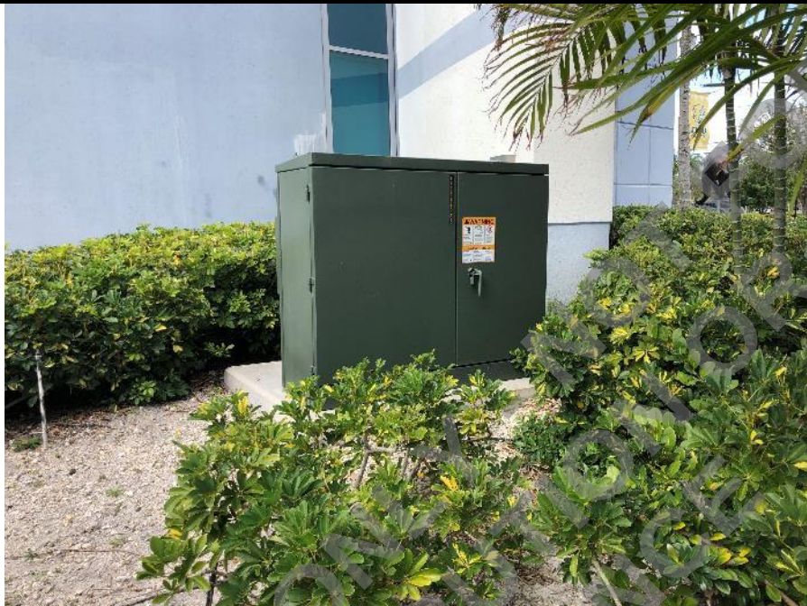
Photo 85: FPL transformer located at east side of property.
