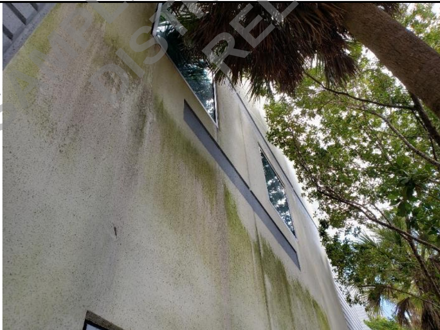
Photo 43: Deteriorating exterior paint and accumulation of a mold-like substance.
