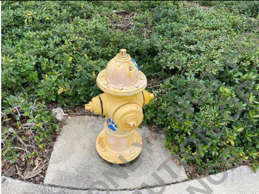
Photo 103: Typical fire hydrant located on the property.
