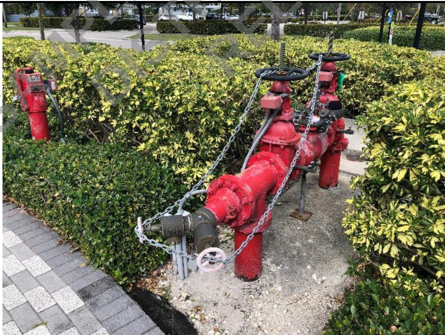
Photo 102: Fire department hose valves located on the property.
