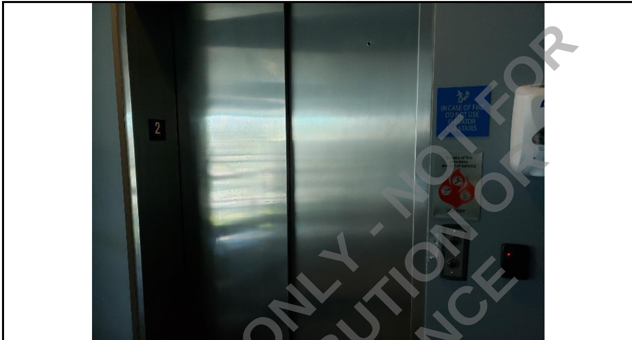
Photo 93: Elevator at lobby mezzanine.
