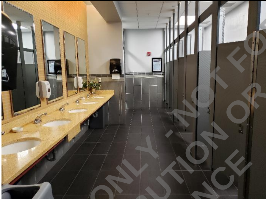
Photo 109: Automatic faucets in restrooms
