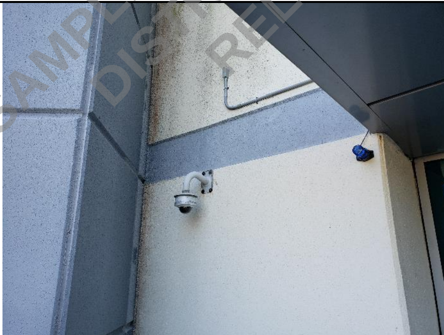
Photo 92: Exterior surveillance cameras mounted throughout building perimeter.
