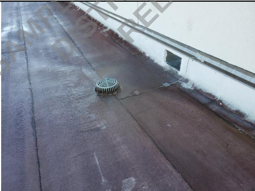
Photo 63: Typical interior drain with overflow scupper.
