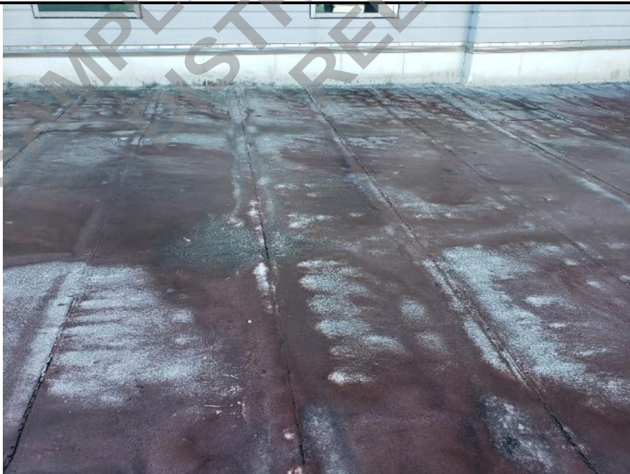
Photo 61: Typical cap sheet weathering observed throughout.
