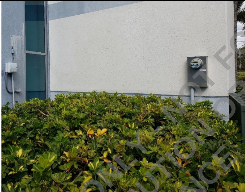
Photo 32: Electrical meter at east side of building.
