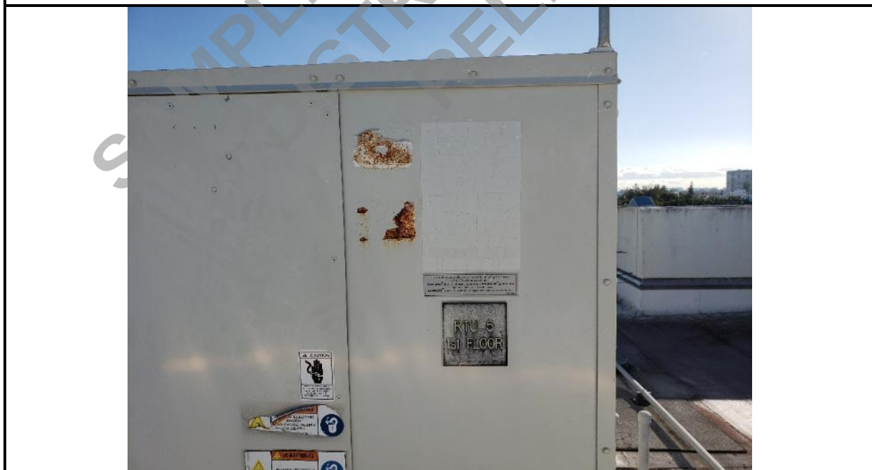
Photo 80: Identification labels faded/not visible on most RTUs.
