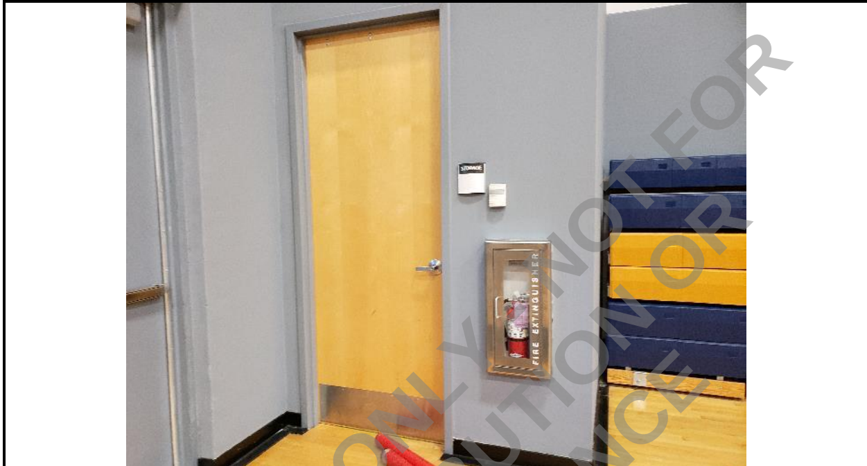
Photo 99: Typical fire extinguisher.
